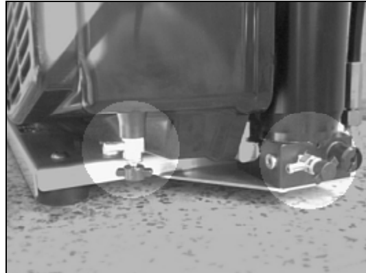
Hand drain valves for the 2nd (left) and 3rd (right) stages
