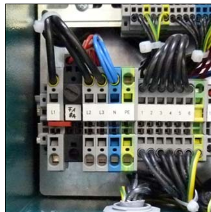
Connection to the switch box
