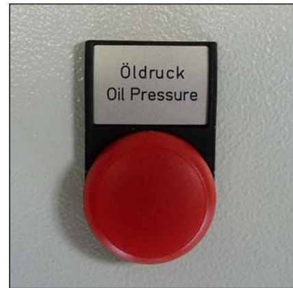
Oil Pressure Monitoring
