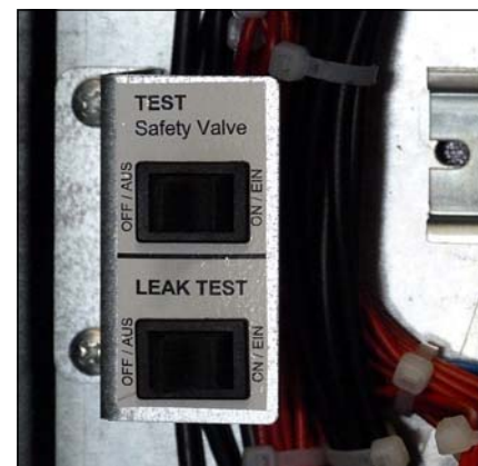
Safety valve test switch (up)
