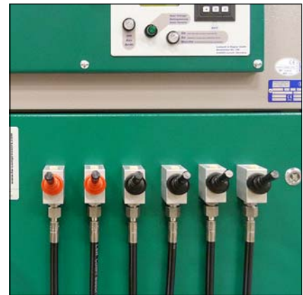
Filling device at the compressor
